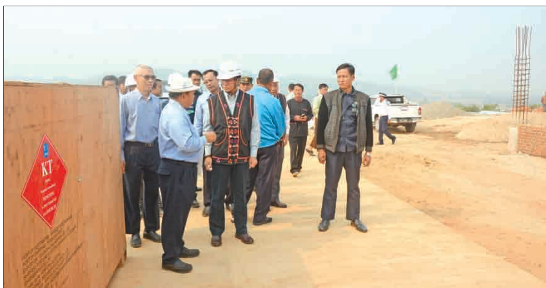
Vice President U Henry Van Thio inspects the construction site of the Kengtung substation in eastern Shan State. PHOTO: MNA
